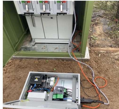
Reliable Communication Infrastructure
