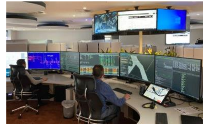
Advanced Distribution Management System
